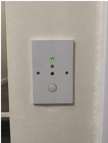
Smoke control override panel, first-floor lobby
